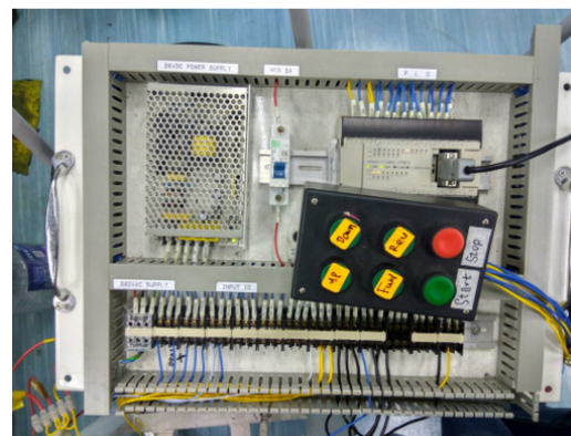
Fig. 10. The PLC Setup and the Controller Buttons
